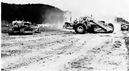
HEAVY EQUIPMENT prepares the base for Ohio University's hard surface runway which has been scheduled for completion the first of October.
